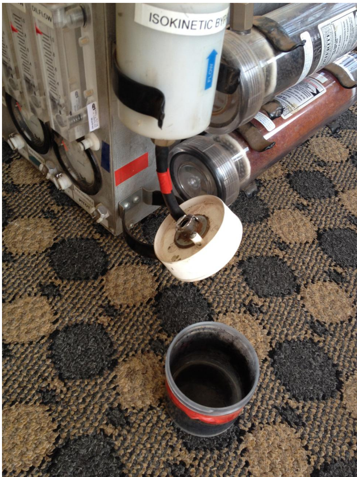
Figure 46: Dump the water trap.
